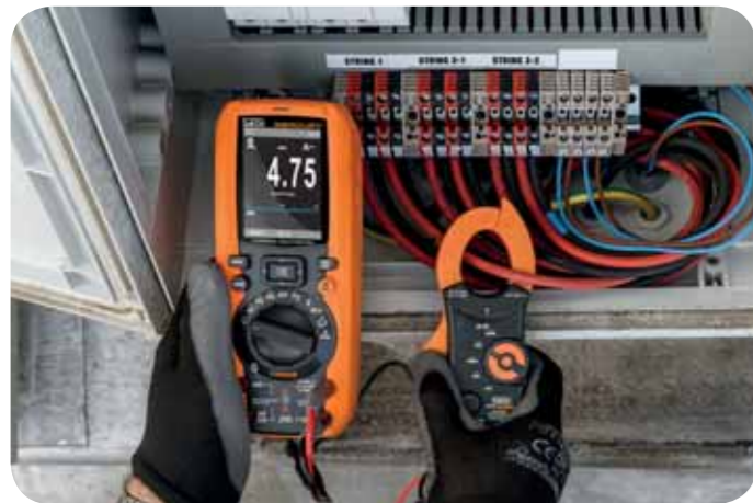
PV string Imp measurement.
