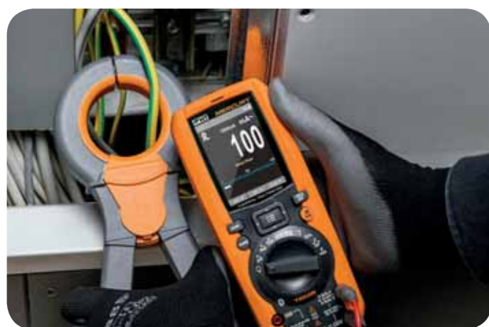
AC leakage measurement.
