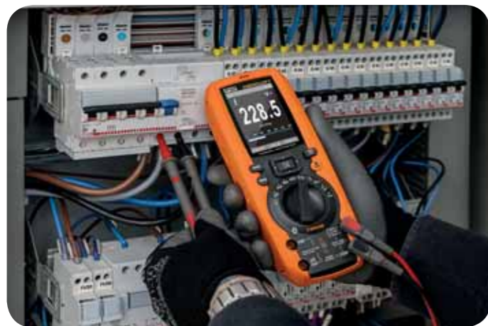
AC voltage measurement.
